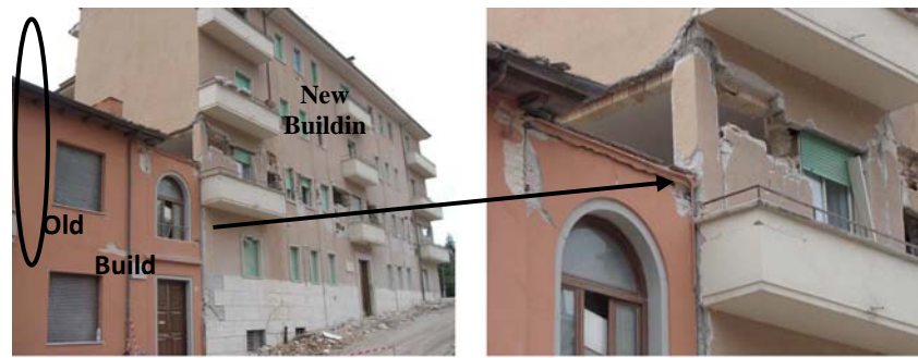
Fig. 2: Pounding between New and Old Building During 6 Apr 2009, L'Aquila Earthquake
