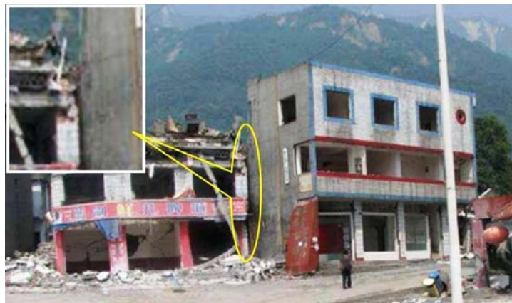
Fig. 1: Pounding Occurred Between Two and Three Storey Structures during 12 Dec 2008, Wenchuan Earthquake (Photo: Khalid M Mosalam)
